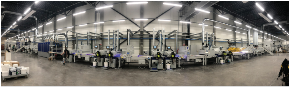
Wide angle view of wood line through fisheye lens, with 7 W-LED systems installed
